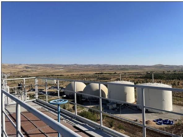
Visit to a sewage plant in Ankara
