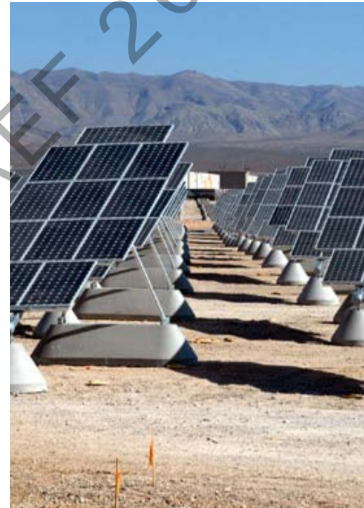
Sunpower silicon panels on trackers
